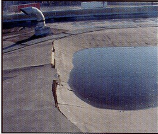
Ponding water obviously caused this collapse, but why did the water pond?
